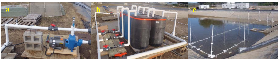
Fig 2: a) pump feeding water from the pond to the CO 2 infusion system, b) the CO 2 infusion system, and c) the discharge manifold.
